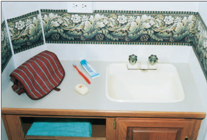
'Small room' wasn't small at all! All sanitary ware is of domestic size (also the plumbing).
