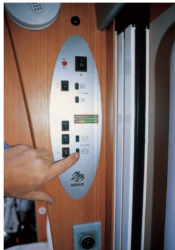
The control panel is just inside the caravan door. Above is a smoke alarm and below the control for the Truma Combi boiler.
