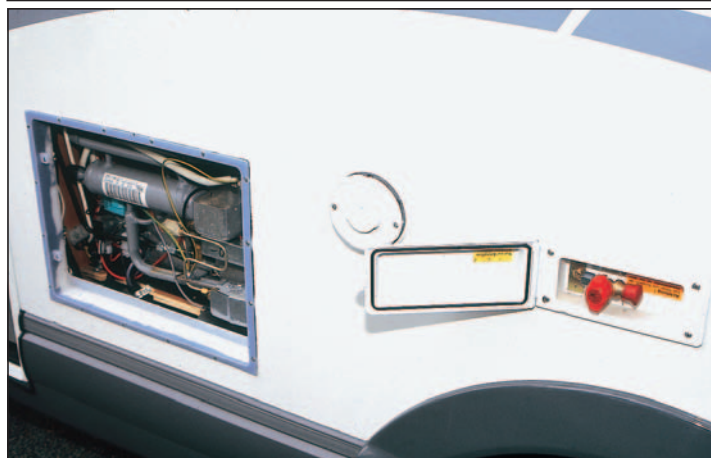
The large, lower fridge vent has been removed to show how easy it will be to service the fridge/freezer. In the middle of the photo is the flue for the Combi boiler and to the right, the external barbecue point.
