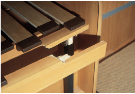
The broken bed structure. All that was holding the whole bed was a half-inch-thick strip of ply. The thicker piece of timber wasn't fixed to the leg. Very strange. A steel frame might be a good idea here.
